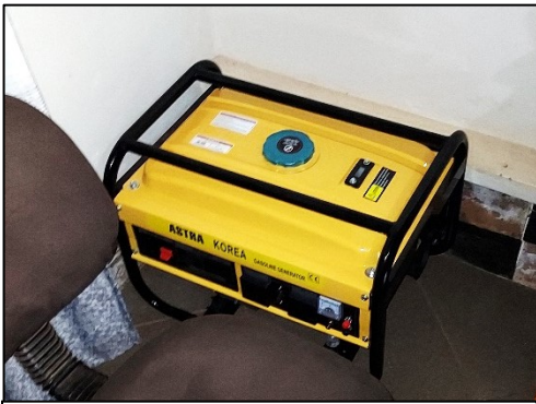
Backup generator for WBS Service Center and GCM offices
